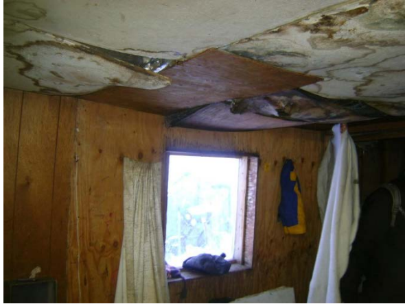
Mold and moisture
